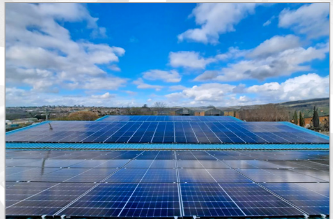
The new solar panels generate over 230,000 Watts Peak.
