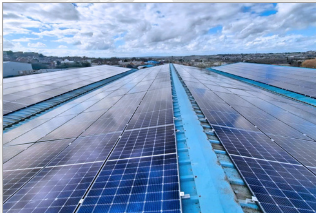
Over 600 solar panels were installed across two sites, generating over 230,000 Watts Peak.
